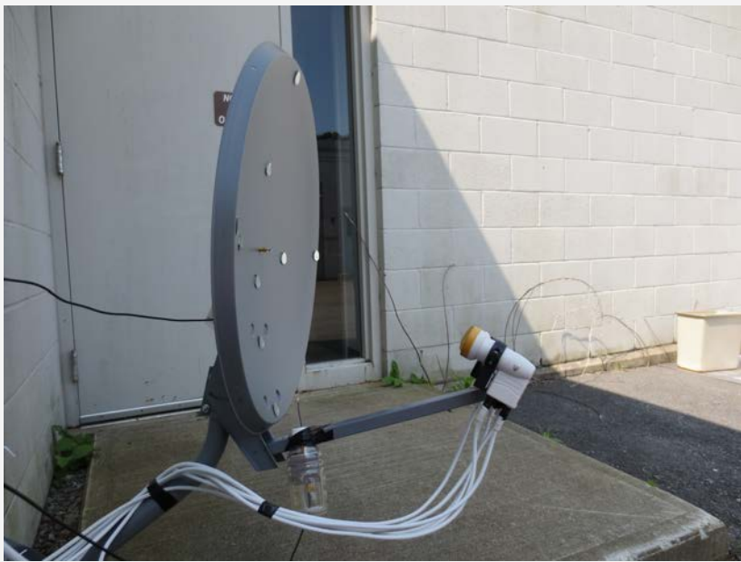
Side view of Antenna and LNB
